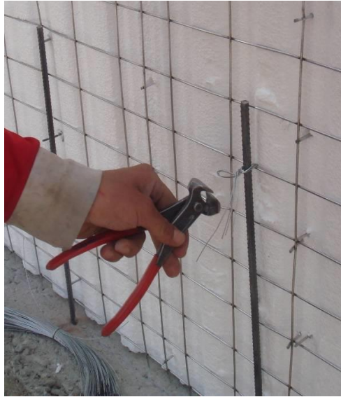
Figure A3.2. Tying panels with corrugated steel installation/foundation by means of wire. Example.
